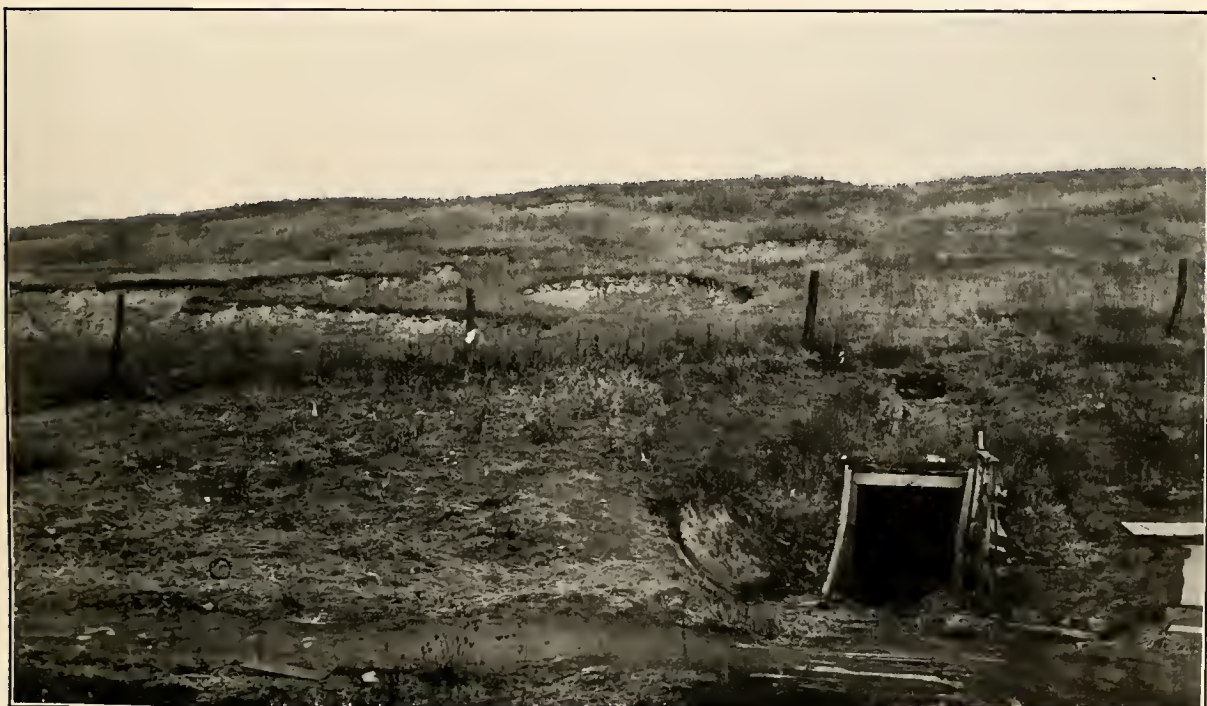
Waste areas in the coal region of southwestern Pennsylvania. Shows the surface caving in where ridges have been tunneled for coal.
